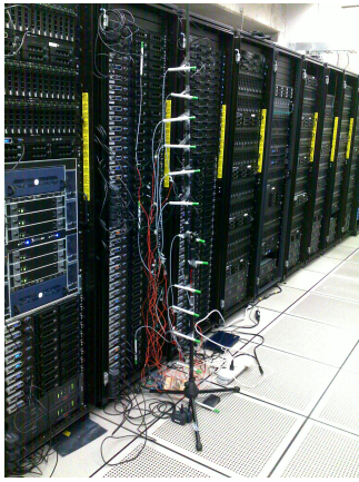
Figure 2: A picture of the air flow sensors setup. We positioned 12 air flow sensors directly above the floor vent at a vertical interval of 5.25’, or every 3U.
